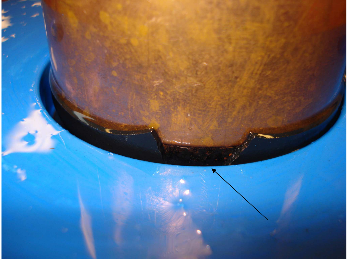
With 'electrolysis insulator'
